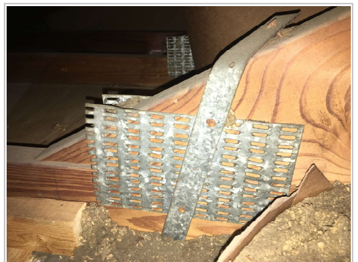
Metal Connectors not Meeting Nail Requirements
